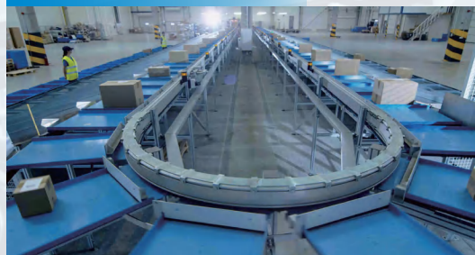
Logistics conveyor line
